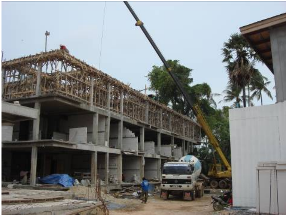
The beams on the third floor of the Apartment building gets concrete
