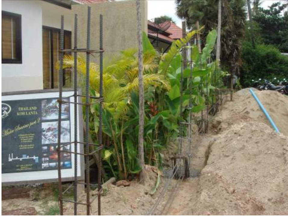
Here is one more picture of the wall to be next to villa C6
