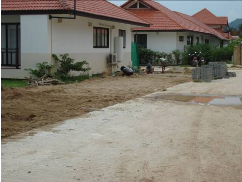
Sometimes the work has to be redone since the workers didn't pack the sand good enough.
