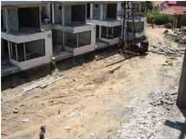
When the piling is finished the glass in the row-house will be installed.
