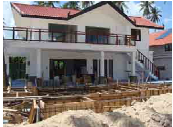
Swimming pool Villa F2 is coming up and the villa is soon to be finished.
