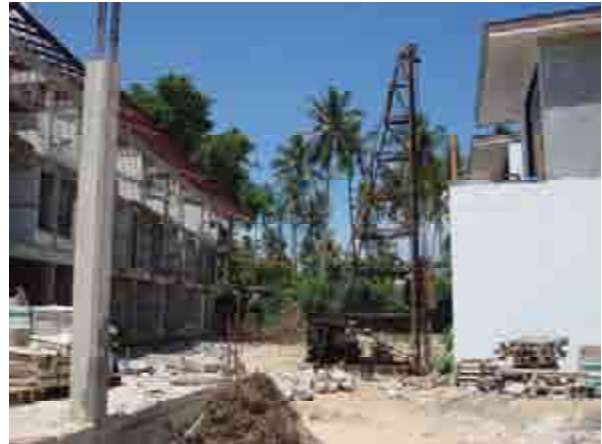
Pilingwork of Sai Naam Swimmingpool. 178 piles are beeing put down in the ground.
