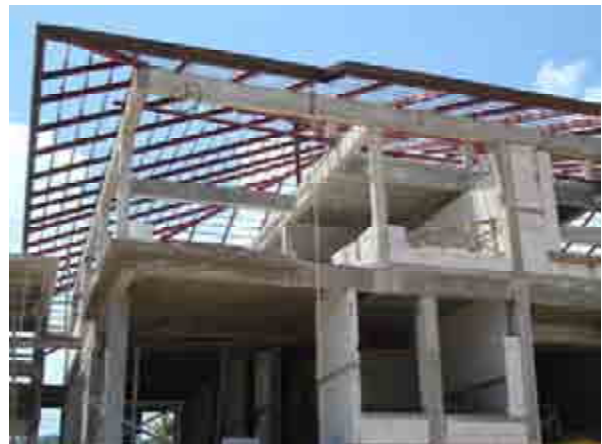
In about a week the Shingle roof will be started to be installed.
