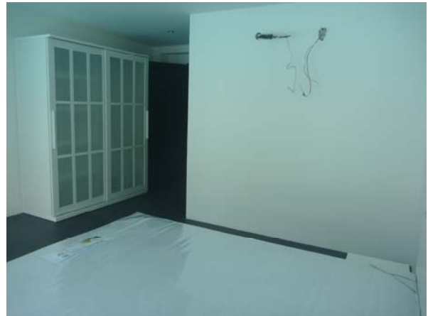
After installation G101
