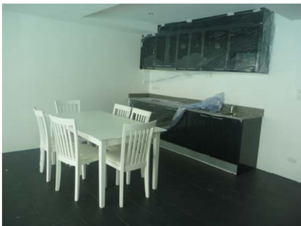
After installation G101
