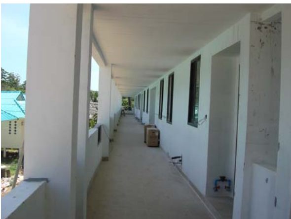
Ac units will soon be installed
