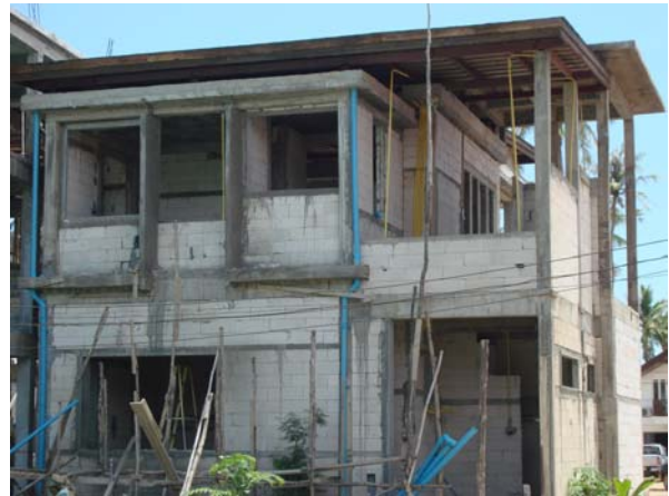
Restaurant building from the back Most 6 pipings are installed
