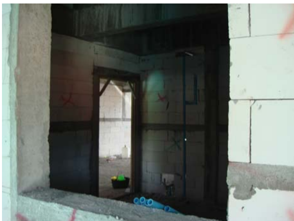
G302 has most of the pipings installed
