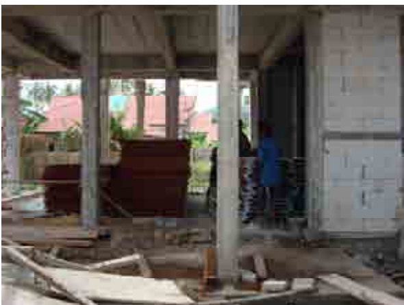
The shingleroof material for the Apartment and Restaurant Buildings has arrived to the site.
