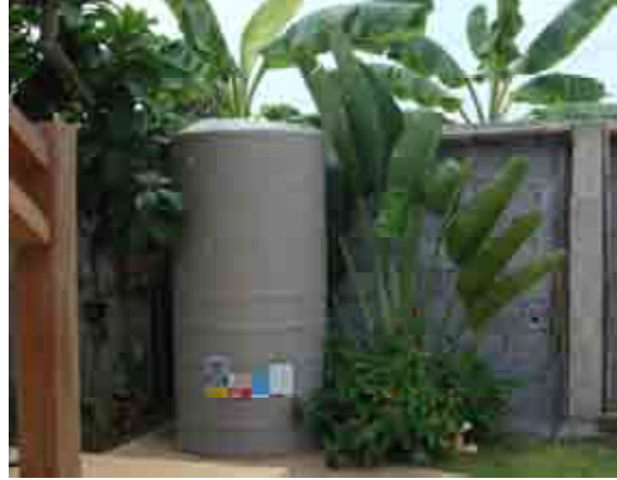
Villa C12 has now installed their own rainwater tank to save the water
