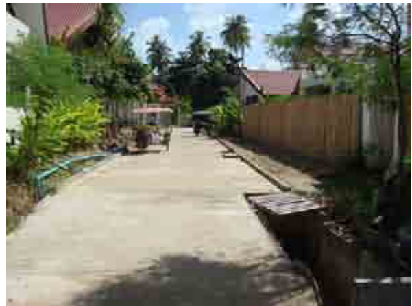
Bic cleaning has been made at Malee Seaview phase 1 The road behind A1-A3
